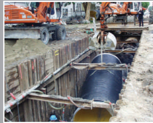
Sewer pipeline DN/ID 2000mm (79")
