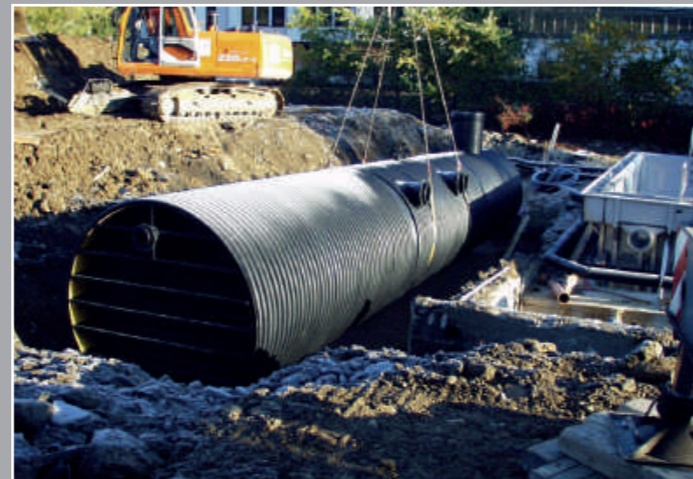
Retention tank of a public swimming pool, DN/ID 3000mm (118")
