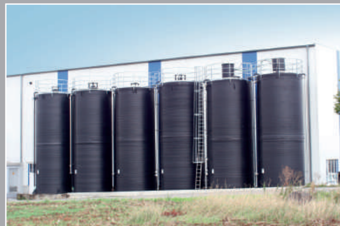
Industrial storage system „silos“
