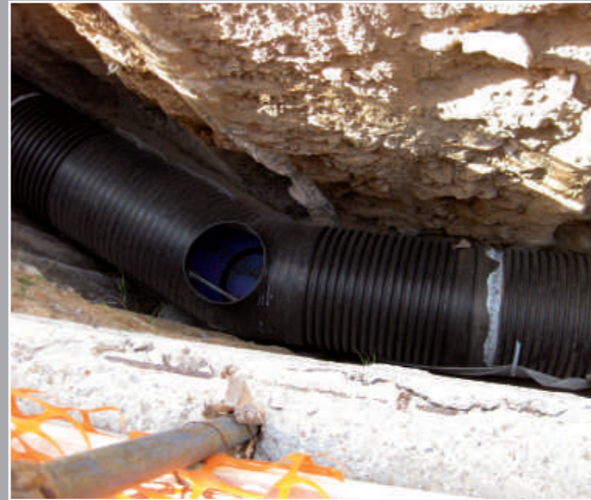
Storm drainage line with integrated manhole
